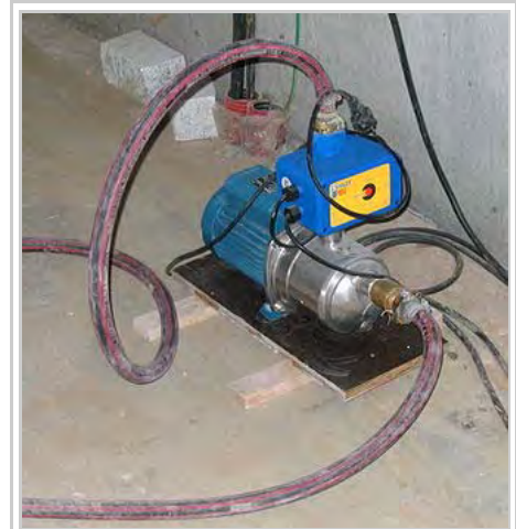
A small, electrically powered pump
