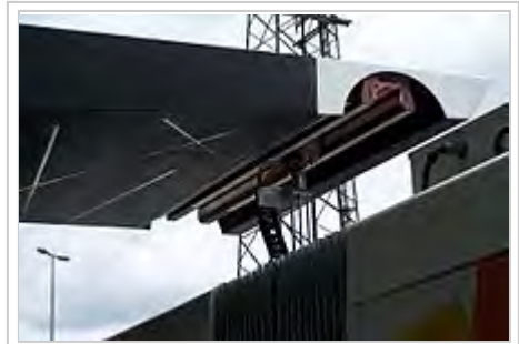
A battery electric bus charging station in Geneva, Swiss
