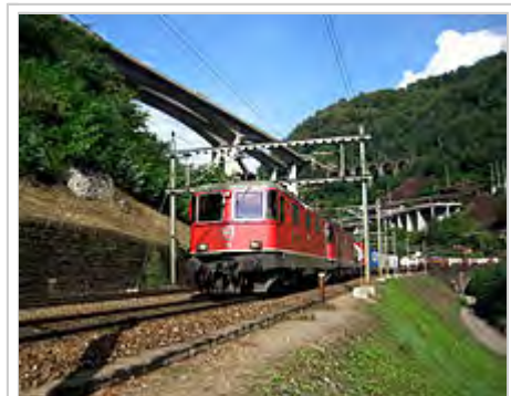
A Swiss Re 420 leads a freight train down the South side of the Gotthard line, which was electrified in 1922. The masts and lines of the catenary can be seen.
