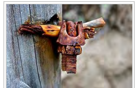
Rusty steel wire rope clamp
