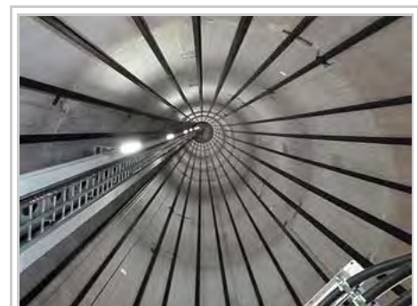
Inside view of a wind turbine tower, showing the wire ropes used as tendons.
