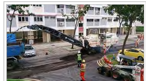
The road surface is removed and a new bitumen layer is added
