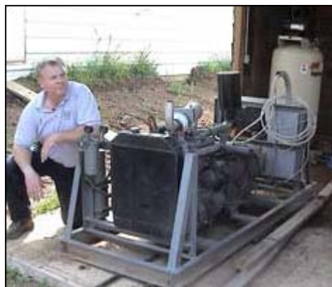
Figure 10: 15 kWe Used Oil Genset (Renewable Oil International)
