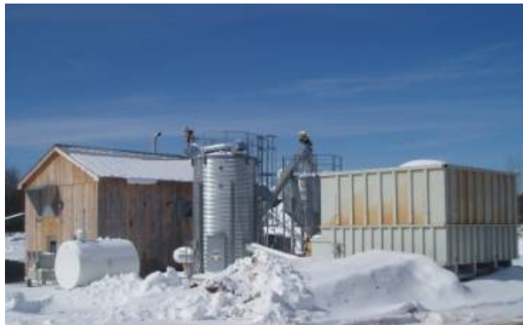
Figure 2: 300 kWe Gasifier at Tallon Lumber, Canaan, Connecticut, 2004
