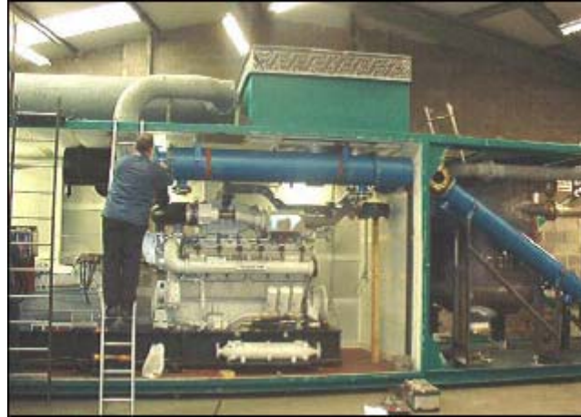
Figure 1: Exus Energy 200 kWe Gasifier and Engine, UK, 2005 (Barker)
