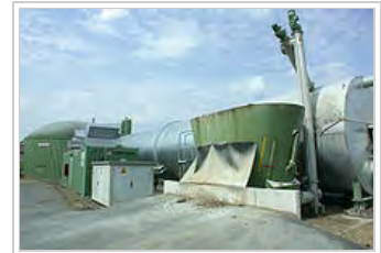
Pipes carrying biogas (foreground), natural gas and condensate
