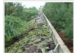
A protective wall built on the shore of the coastal town of Kalpakkam, in aftermath of the 2004 Indian Ocean earthquake.
