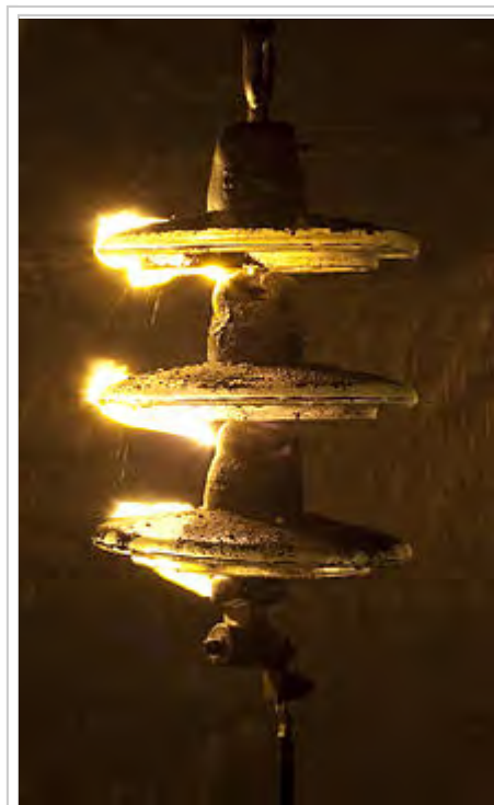
Electrical insulator flashover caused by volcanic ash contamination.
