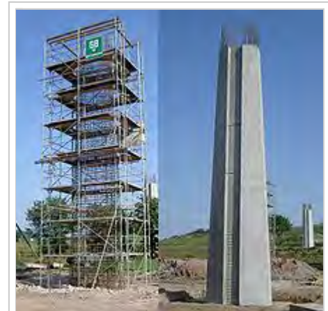
A heavy reinforced concrete column, seen before and after the concrete has been cast in place around the rebar cage.
