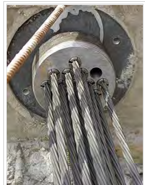
Post-tensioned tendon anchorage. Four-piece "lock-off" wedges are visible holding each strand
