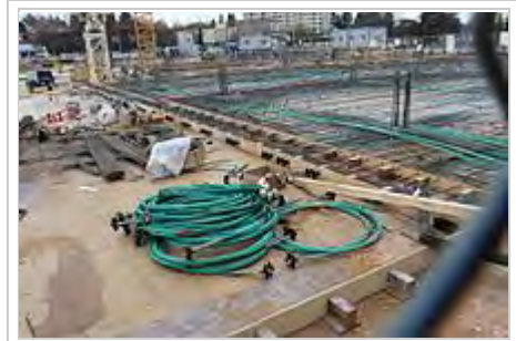
Unbonded slab post-tensioning. Installed strands and edge-anchors are visible, along with prefabricated coiled strands for the next pour
