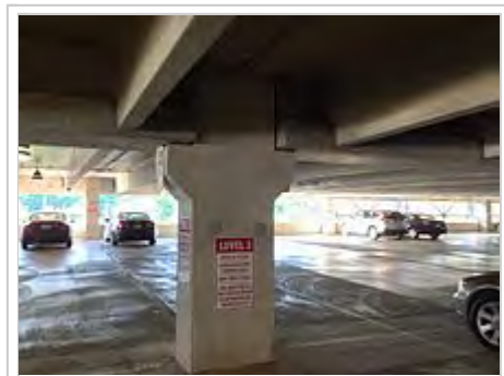
Precast parking structure showing an interior column, girders and double-tee structural floors. The two gray circles are covers to close the lifting anchor holes.
