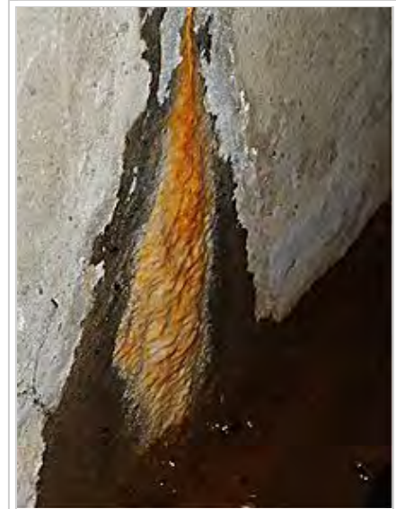
Calthemite flowstone stained orange from rusting reinforcing (iron oxide) being deposited along with calcium carbonate
