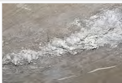
Example of secondary efflorescence in parking garage exposed to diluted road salt from vehicles entering the garage during winter.
