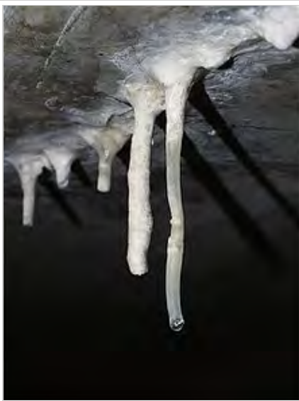
Stalactites growing beneath a concrete structure as a result of calcium hydroxide being leached from concrete and deposited as calcium carbonate to create calthemite forms beneath structure
