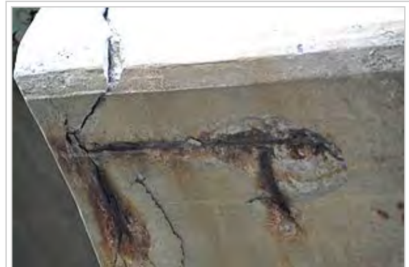
Degraded concrete and rusted, exposed rebar on Welland River bridge of the Queen Elizabeth Way in Niagara Falls, Ontario.
