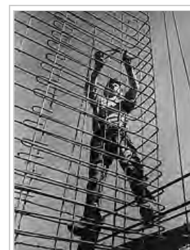
Constructing a rebar cage. This cage will be permanently embedded in poured concrete to create a reinforced concrete structure.
