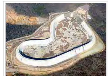
Aerial photo of reconstruction at Taum Sauk (Missouri) pumped storage facility in late November, 2009. After the original reservoir failed, the new reservoir was made of roller-compacted concrete.
