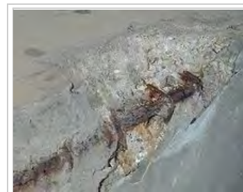
Concrete spalling caused by the corrosion of rebar
